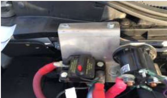
Typical Ford Installation on Passenger Side of Engine Compartment 2017 - Current
